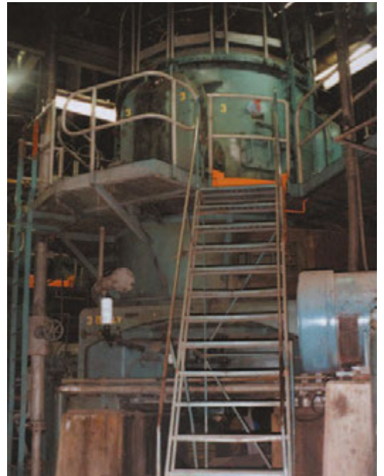
Combustion Engineering 783RP Bowl-Mill Coal Pulverizer.
